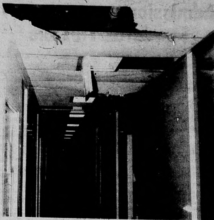
Rain water damages the 5th floor of Matheson Hall.
